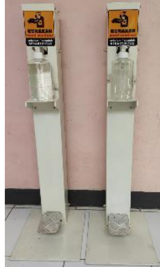
Gambar 6a. Instalasi Portable Sanitizer
